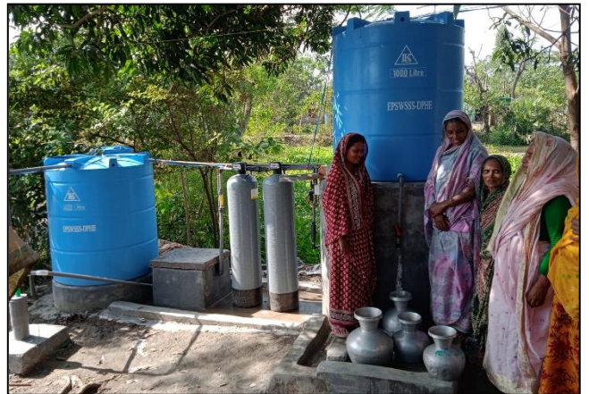
Pic- AIRU installation by DPHE at Khagail village in Horidaspur Union
